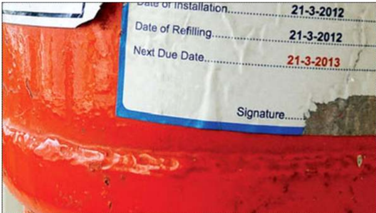
Fig 18.4.1.3 Know the refill date on the fire extinguisher
